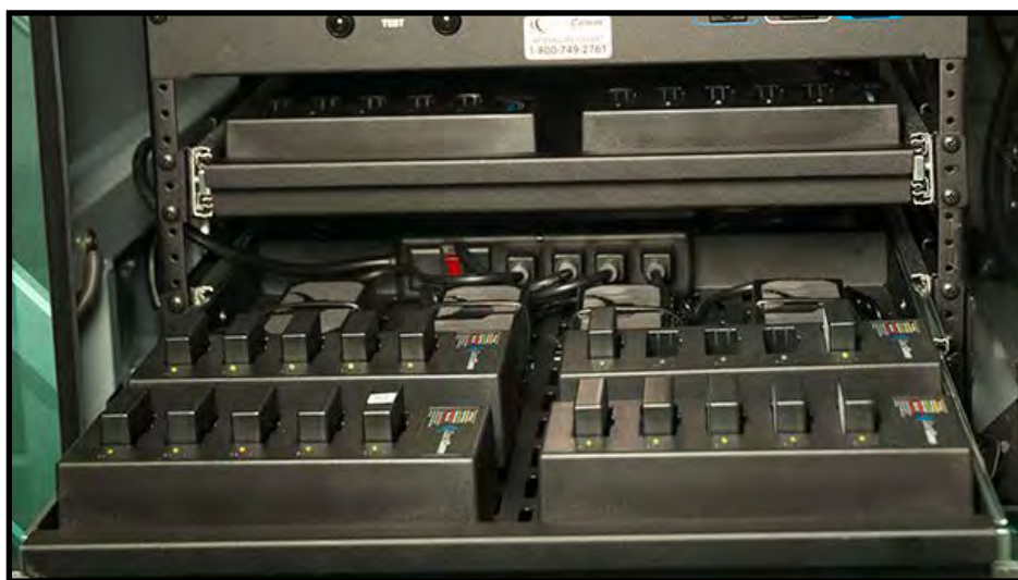
Figure 53: 5-Bay Battery Chargers
