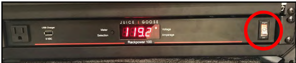
Figure 38: AC Power Distribution Unit Switch
